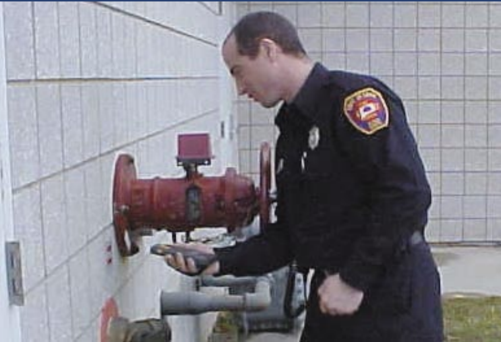
UConn Firefighter Paul Burton conducts monthly inspection of sprinkler control valves.
