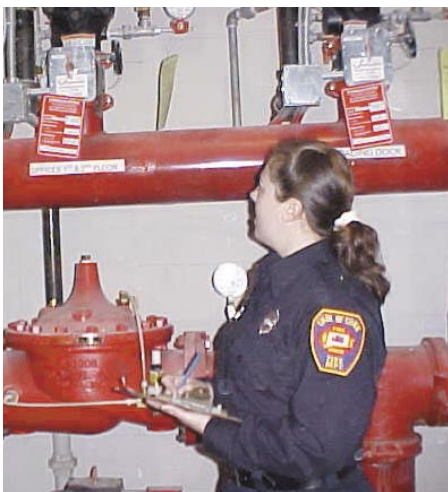
Heidi Vasseur, a member of UConn’s fire department, checks to see if control valves are in “open” or “locked” position.
